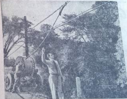
Construction program the biggest in our history. Our manufacturing and supply unit, the Western Electric Company, turned out switchboards, cables and other com- plicated apparatus in tremendous volume. 1,000,000 miles of wire in new cables were placed in service so that more telephones could be connected.
